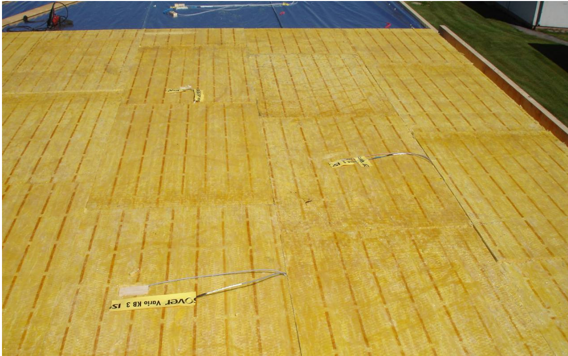
Figure 9: Installation of the exterior sensors (on top of the insulation layer) for RH and temperature measurement.
