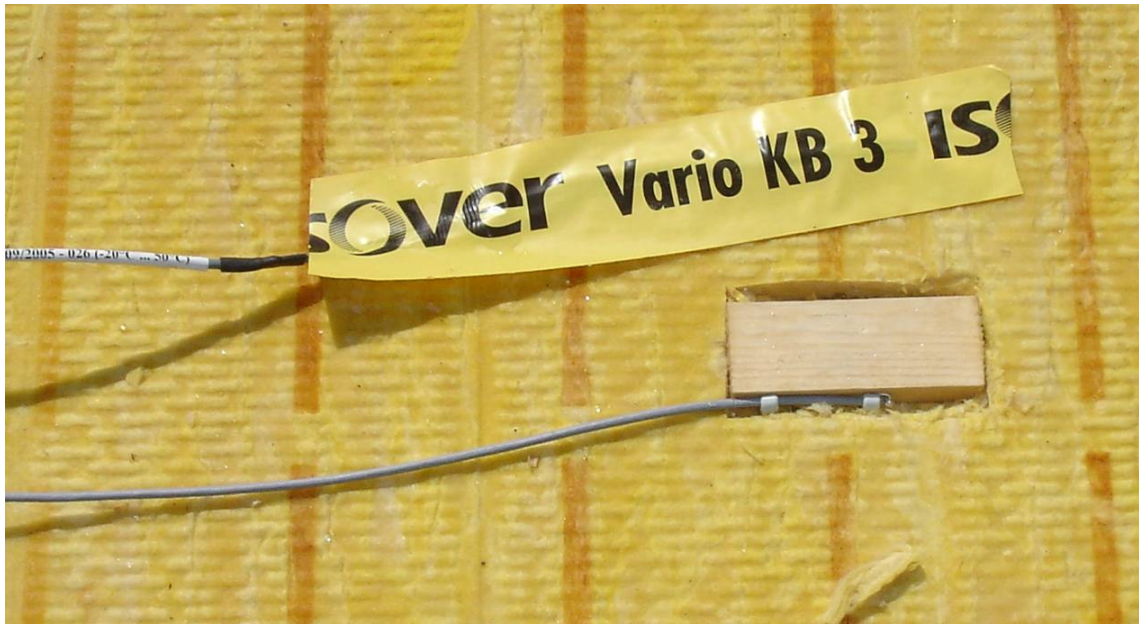
Figure 11: Close look at the wooden cubes with electrical resistance moisture sensors next to a PT100 on top of the insulation layer.
