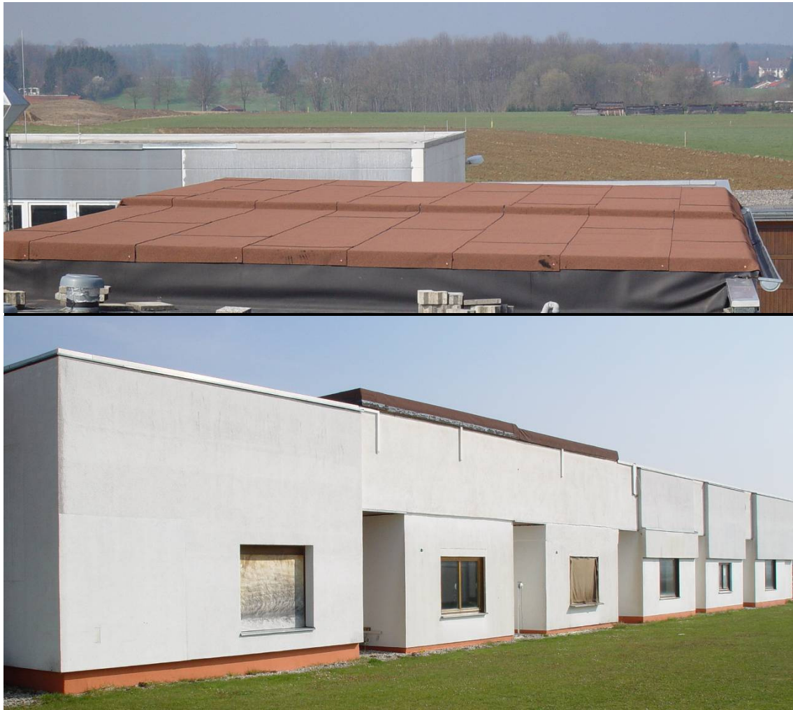
Figure 14: View of the finished flat roof sections from the top and from the south side of the test building.
