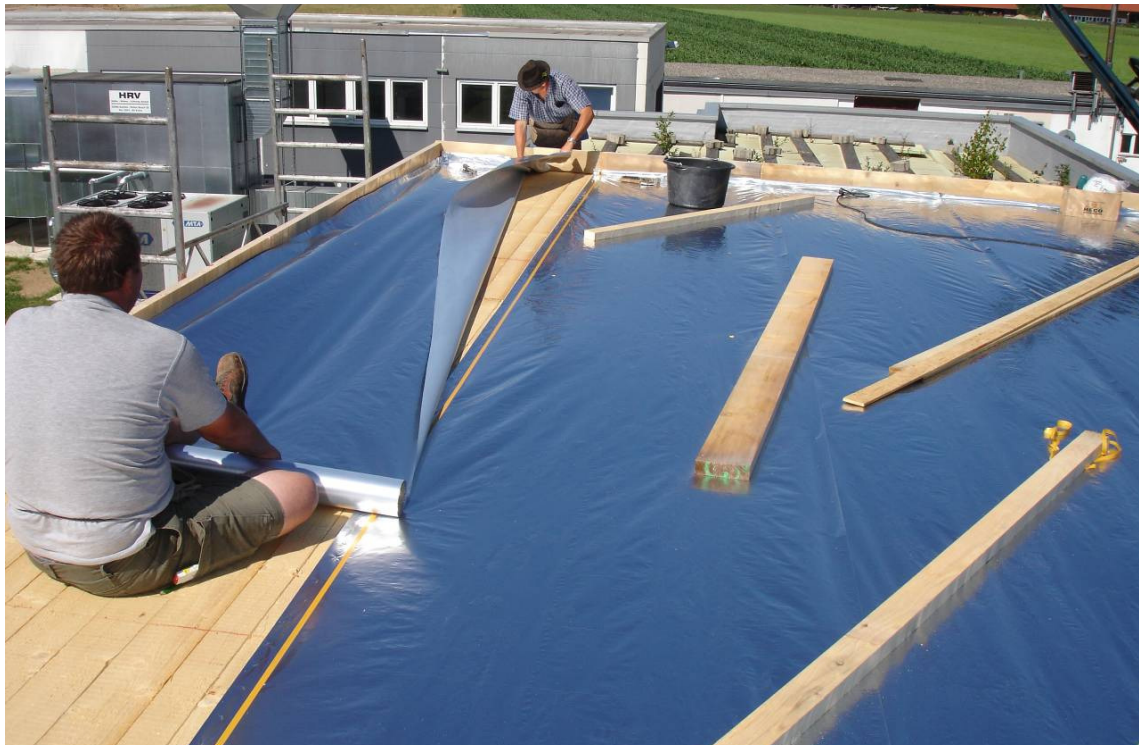
Figure 5: Airtight application of the aluminium vapour barrier on the wooden sheathing over the attic space.
