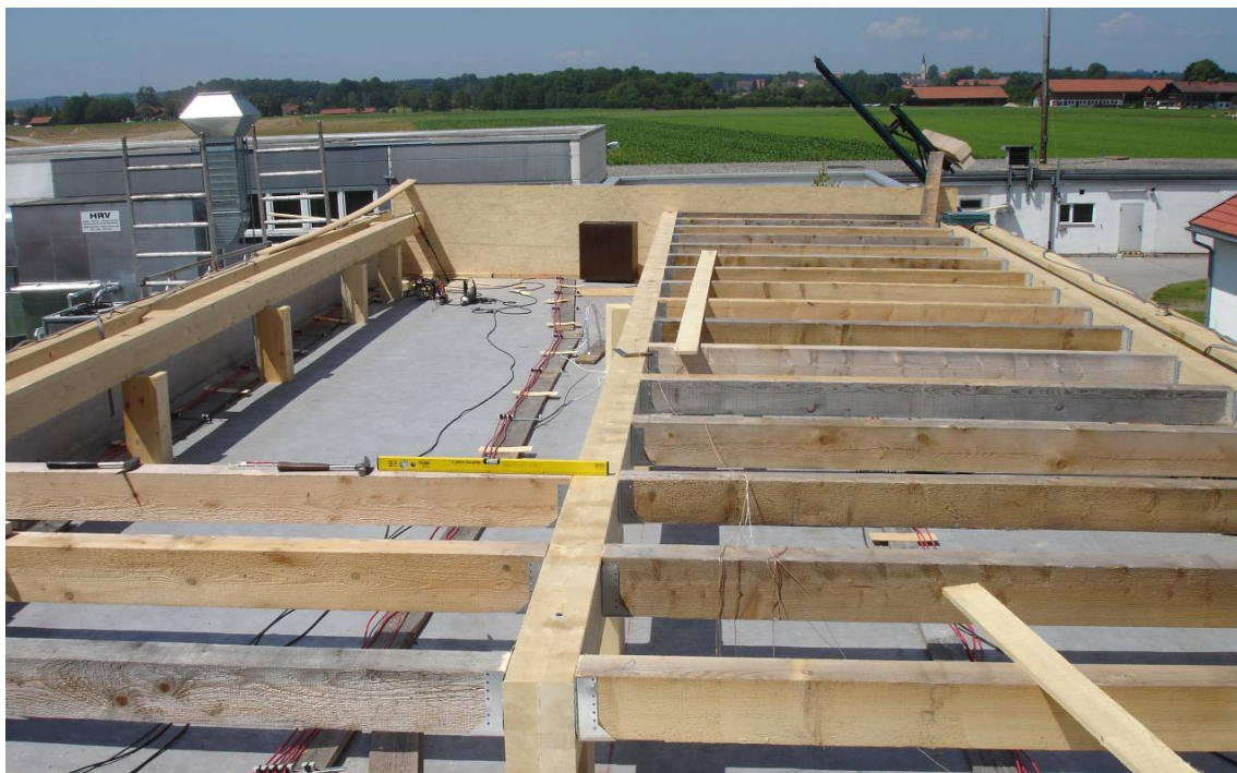
Figure 4: Installation of electrical wire heating and preparation of the load bearing roof structure above the attic space.
